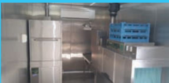
Rack conveyor dishwasher with a 6KW drier, and a pot washer
