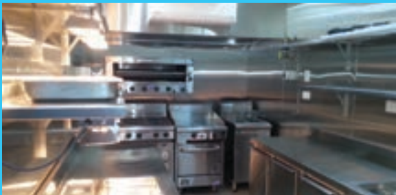
Complete commercial kitchen
